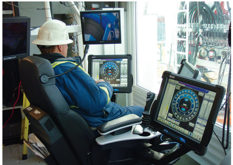
With multiple screens and touch and joystick controls, the PRECISE system enables full control of drilling functions from a single source.
