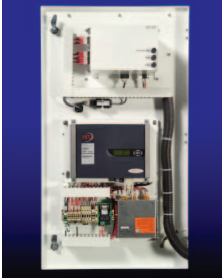
Internal view of the FixStar model 3900's low-voltage compartment with optional espWatcher* transceiver.
