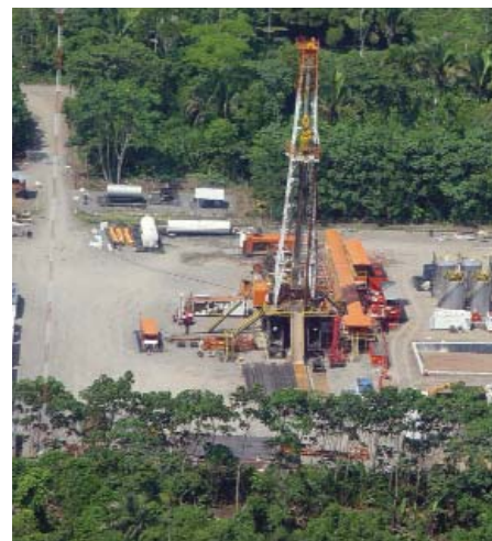
Figure 5. Located in the lush tropical forests of northeastern Ecuador, the clean, compact drillsites of Block 18 are examples of Petrobras' strict environmental stewardship.
