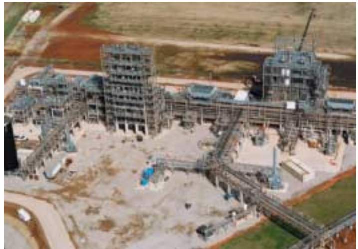
^ The ConocoPhillips GTL demonstration plant in Ponca City, Oklahoma, USA. The plant was completed in March 2003, and is designed to convert 4 MMcf [114,600 m 3 ] per day of natural gas into 400 B/D [64 m 3 /d] of sulfur-free diesel and naphtha. (Photograph copyright of ConocoPhillips.)
