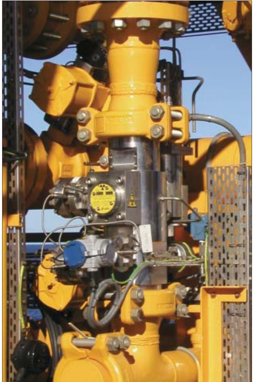
The Schlumberger PhaseWatcher installed on an unmanned platform offshore Australia.
