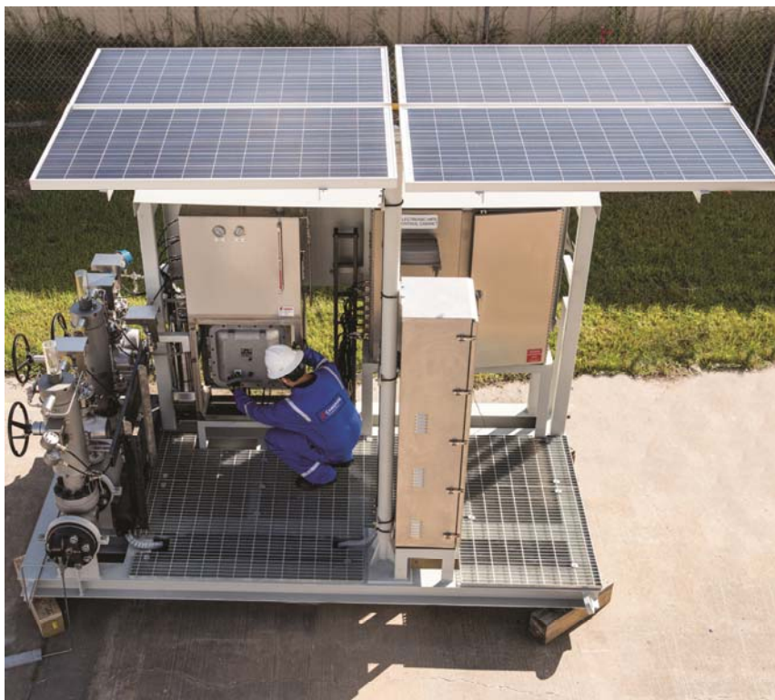
A Schlumberger expert prepares the HIPPS prior to testing. (Image courtesy of Schlumberger)
