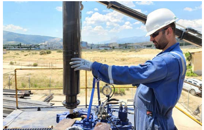
REDA Thermal ESP was run into a geothermal well in Kizildere Field to improve flow rate.
