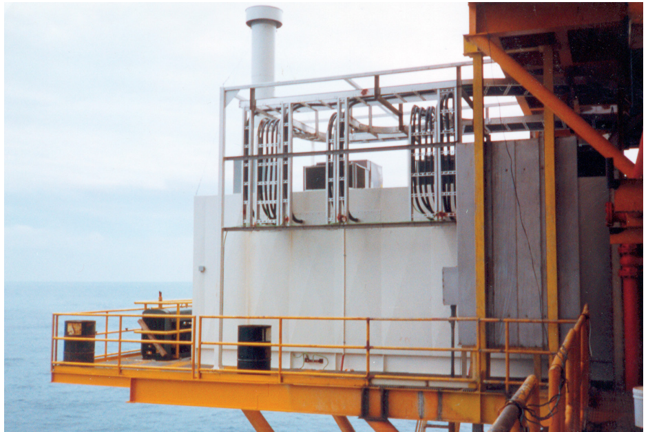
An offshore 800-kVA at 480 V VSD module for the Gulf of Mexico.
