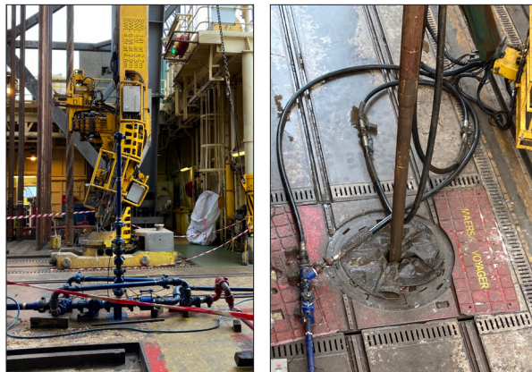
(Left) Side view of 3-in foam cross manifold coupled with two parallel 2-in lines, which permitted high job flow rates. (Right) An overhead view of a T junction that permits the use of two parallel lines. This method makes it possible to pump at higher flow rates.
