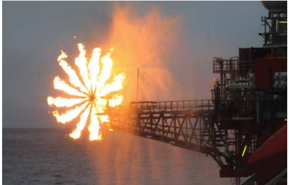
EverGreen burner and water-cooling wall burning hydrocarbons during the flow period of the horizontal well test.
