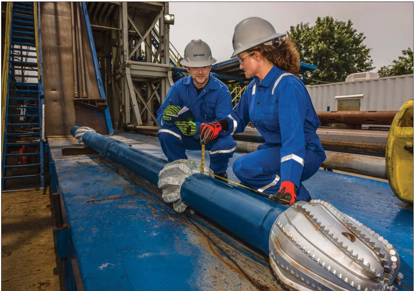
^ Making the grade. Every component is measured and calipered before going in the hole. Once the milling assembly is retrieved, each mill is graded for wear. The lead mill ( foreground ) is designed to initiate the cutout and mill the window as it slides down the whipstock. It also drills the rathole. The follow mill ( middle ) engages the casing and elongates the window. The dress mill ( background ) removes rough edges around the window.
