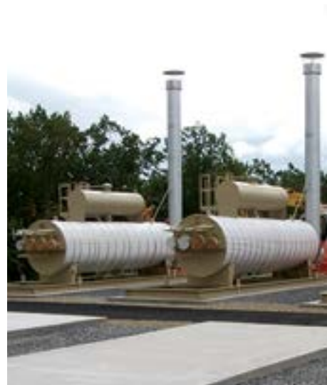
Water bath heaters.
