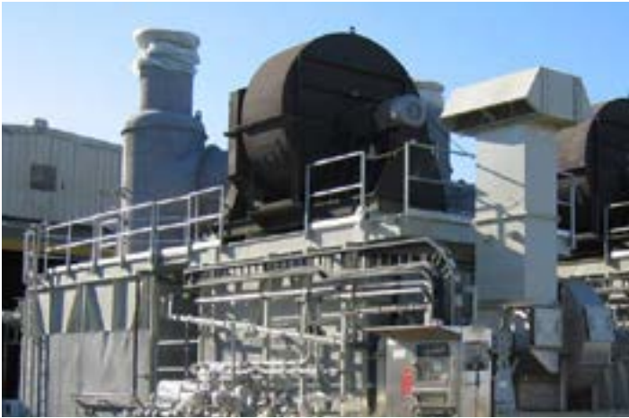
NATCO CHF controlled-heat flux heater with 1,000-degF process outlet temperature capability.
