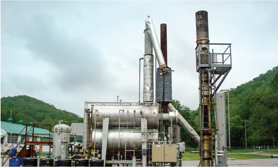
NATCO SHV Flare emission control system.
