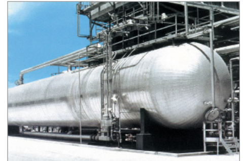
PETRECO BILECTRIC AC desalter.
