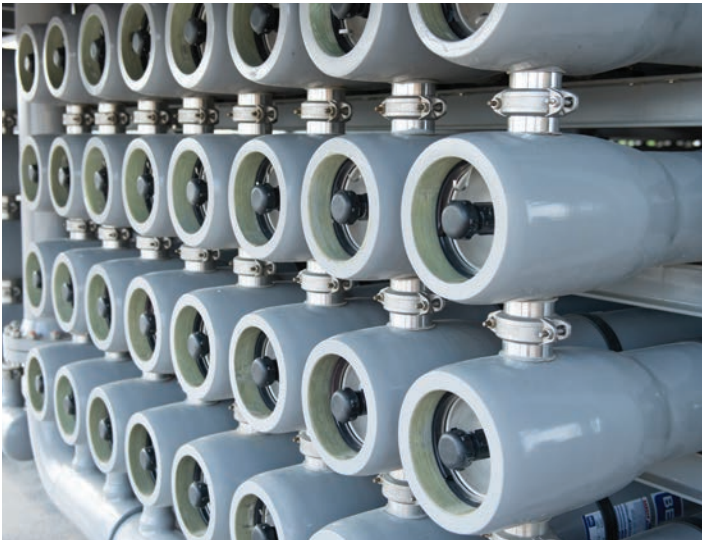
End view of membrane pressure vessels.
