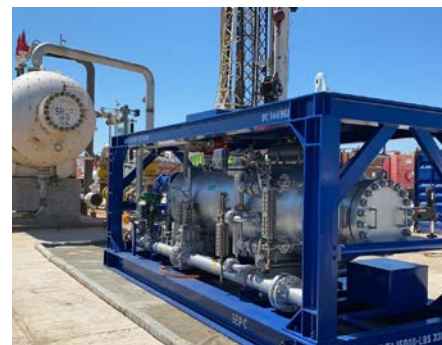
The PEMEX legacy separator was augmented by this rapid-response, fit-for-basin separator provided by Production ExPRESS solutions.
