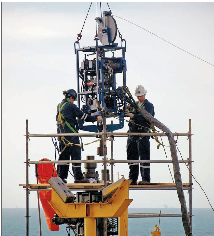
BJ Services crew members prepare to run a capillary string for an InjectSafe system installation in the Gulf of Mexico.
