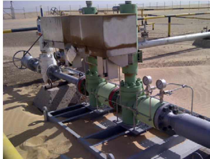
Mechanical HIPPS skid in Saudi Arabia.
