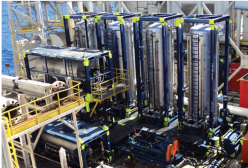
This configuration offshore Brazil uses four surge tanks for greater storage capacity to meet test requirements.
