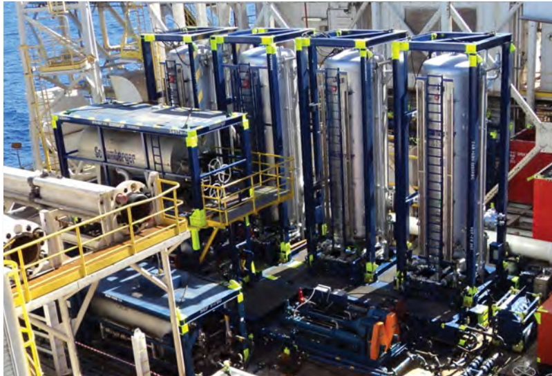
This configuration offshore Brazil uses four surge tanks for greater storage capacity to meet test requirements.
