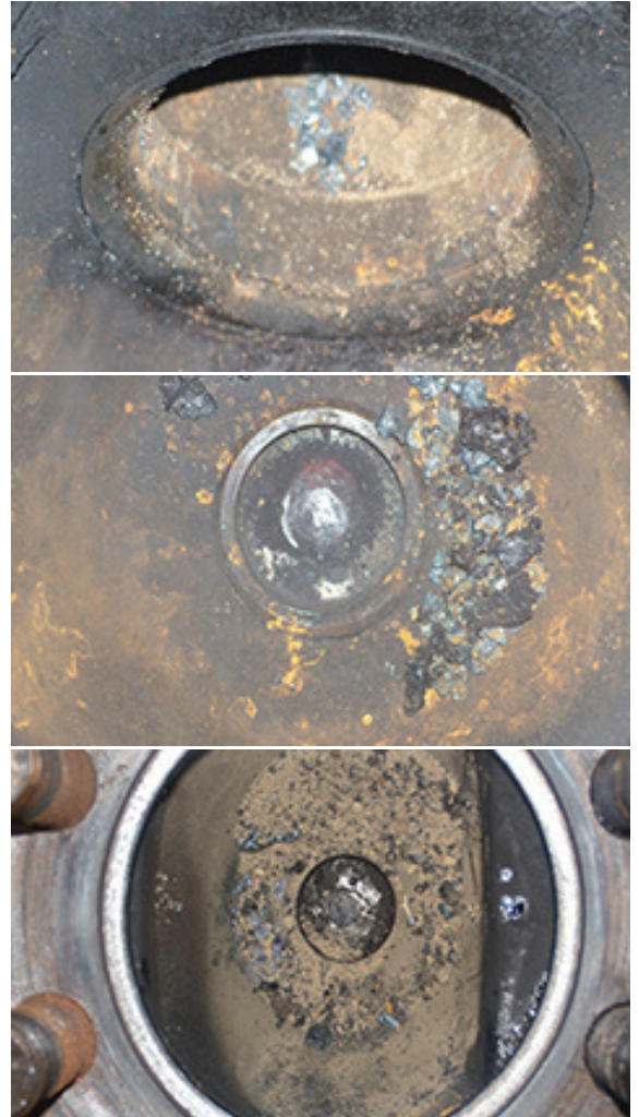
Examples of damage caused by weld slag during construction.
