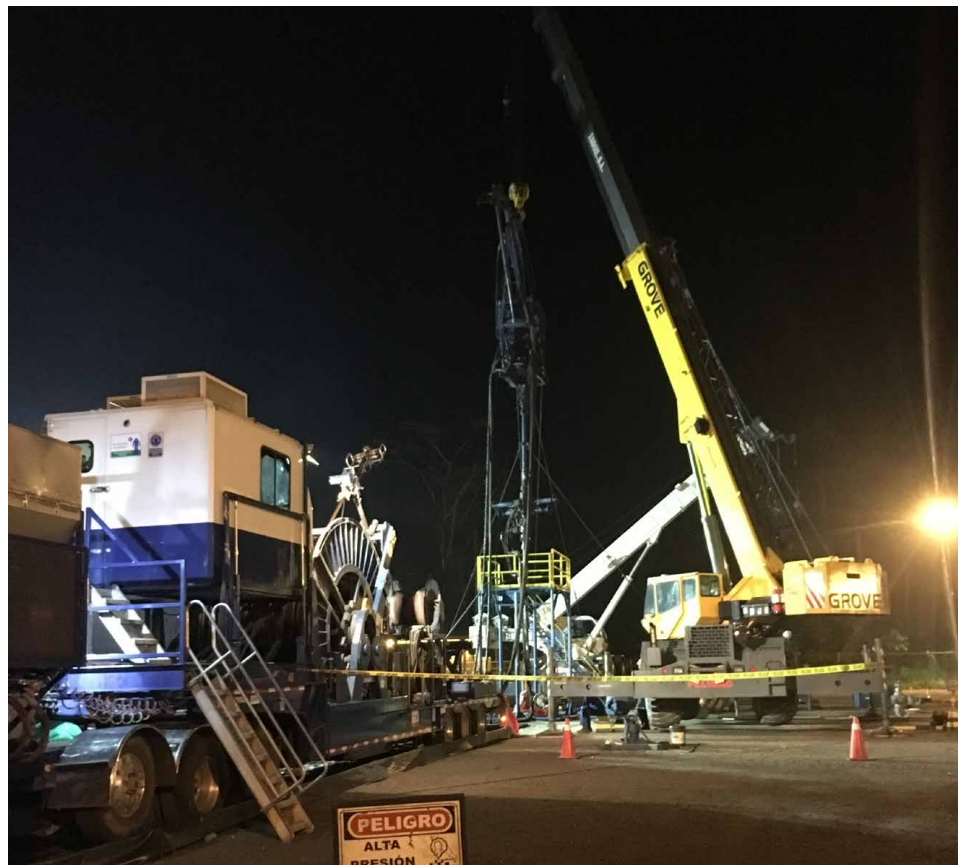
The ZEiTECS Shuttle system enabled rapid ESP replacement without a workover rig, reducing costs and eliminating more than 5 days of deferred production.
